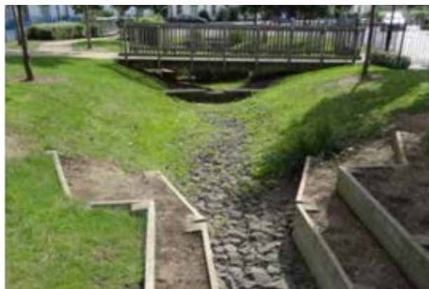
Image below: Demonstrates impact of erosion
