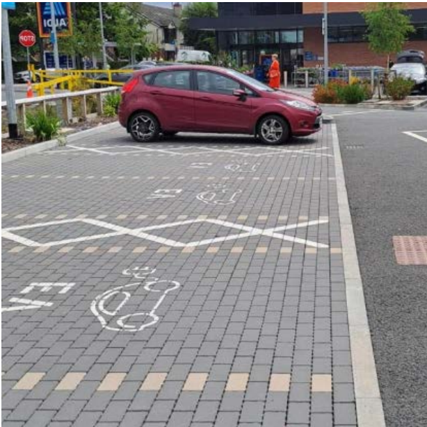
Image above: Concrete Block Permeable Paving - Aldi Stores, Main Street, Newbridge
